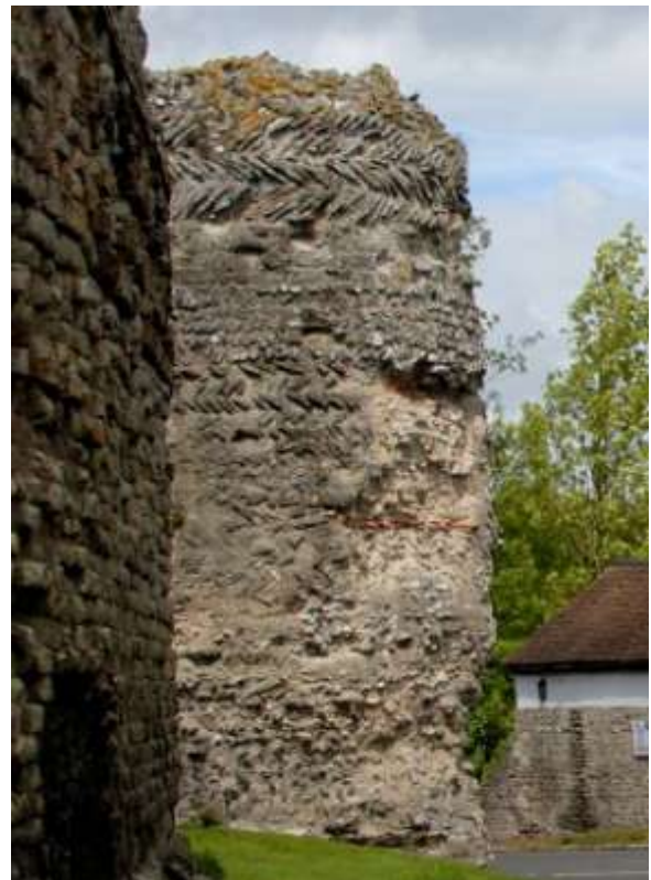
Fig. 10. Roman bastion north of the east gate showing repairs, probably of the late 11 th century, in herringbone-coursed rubble.
