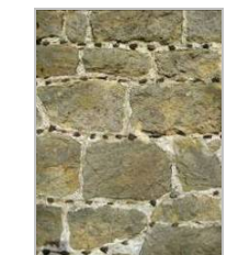
Ironstone galleting in sandstone wall
