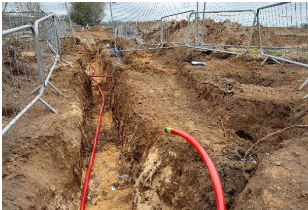
Figure 1: New HV Cable
