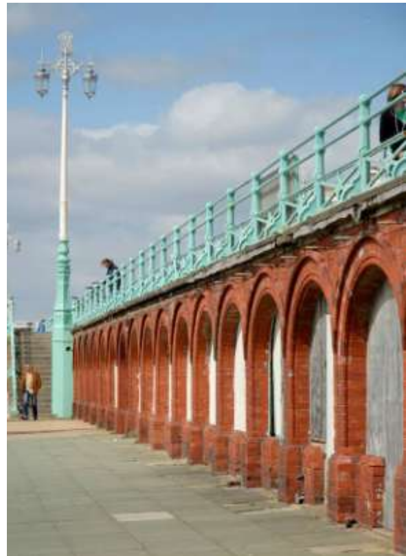
Fig. 59. Lower Esplanade, King's Road: arches, railings and lampposts 1883-7, lights 1980s replicas of 1930s originals.
